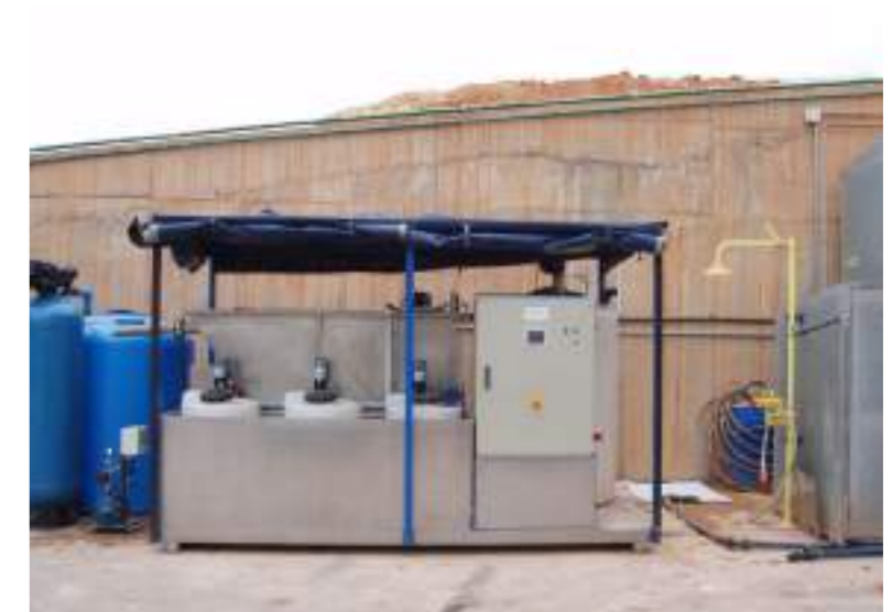
Portable industrial wastewater treatment plant. Flow 2 m 3 /h.
