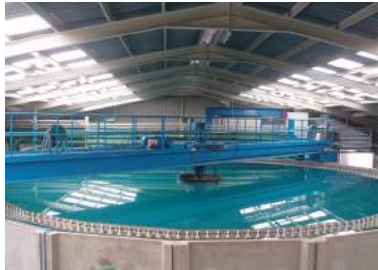
Industrial wastewater treatment plant. Flow 300 m 3 /h.
