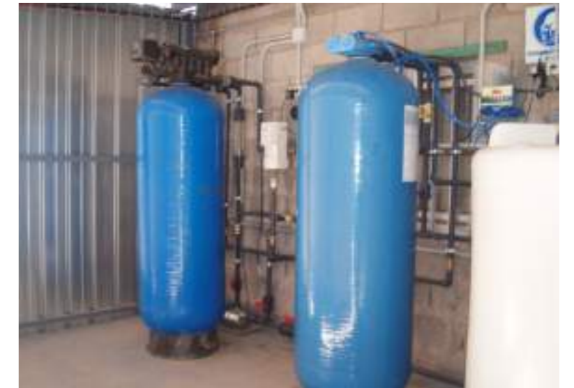
Boron removal treatment. Flow 3 m 3 /h.
