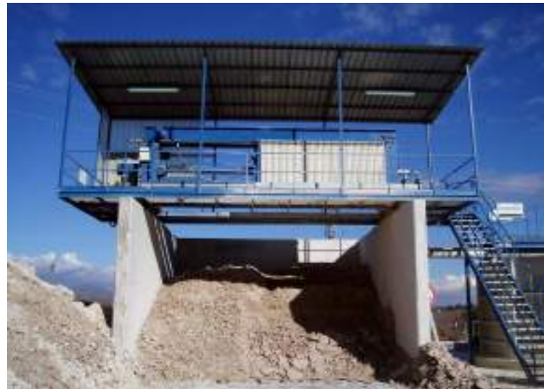
Filter press for sludge dewatering.
