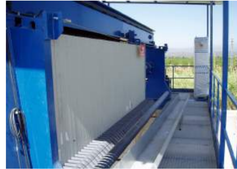
Filter press for sludge dewatering.
