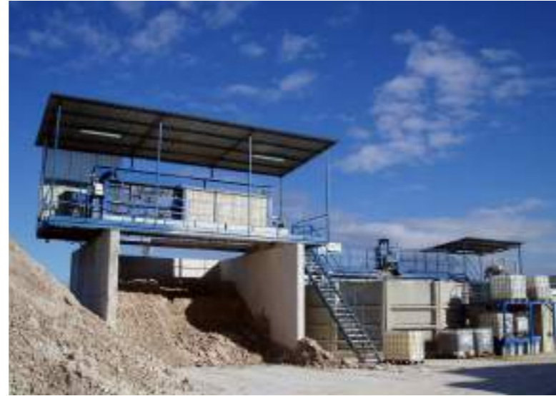
Industrial wastewater treatment plant. Flow 80 m 3 /h.
