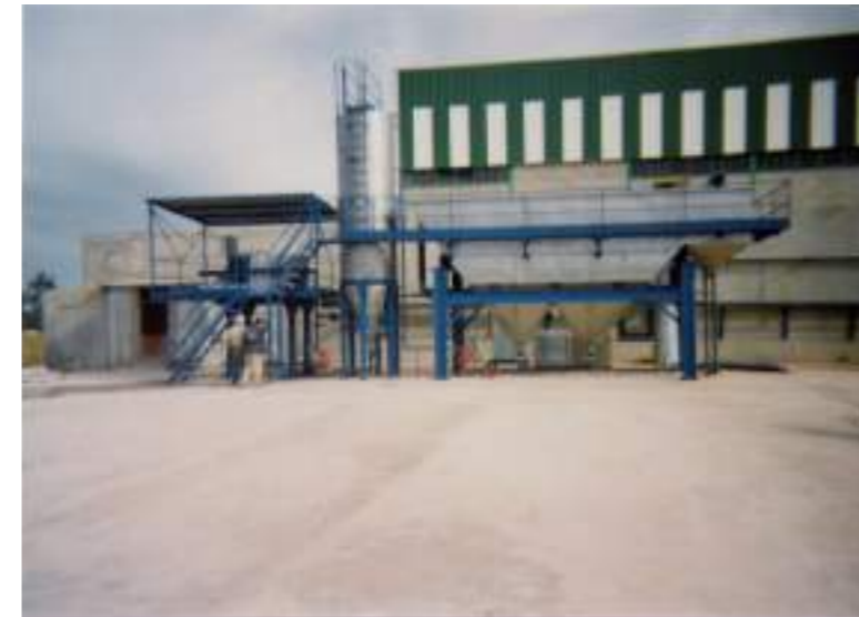
Industrial wastewater treatment plant. Flow 150 m 3 /h.
