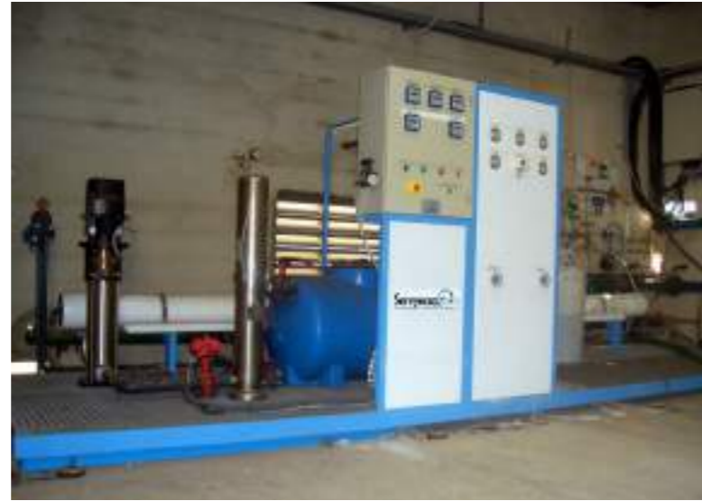
Reverse osmosis. Flow 100 m 3 /day.
