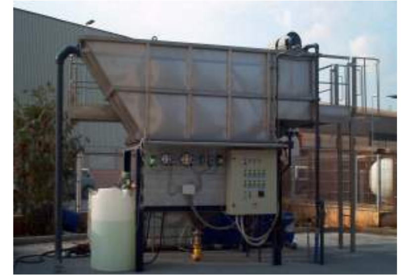
Industrial wastewater treatment plant. Flow 5 m 3 /h.
