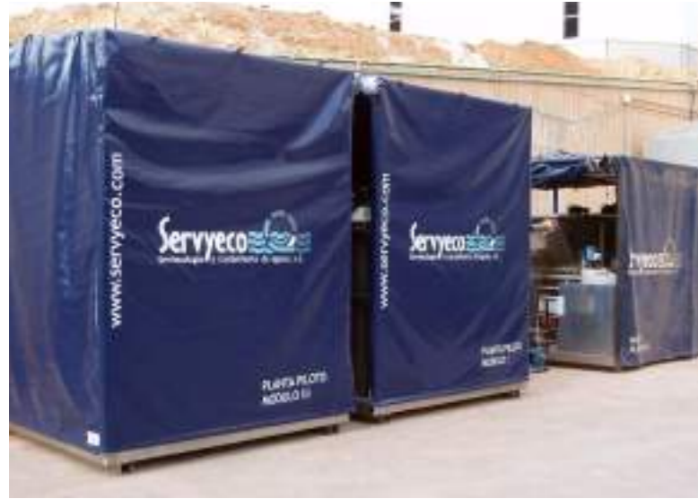
Portable modular demonstration pilot plant. Flow 2 m 3 /hora.
