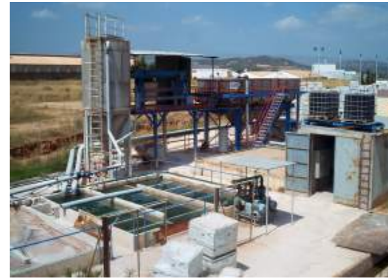
Industrial wastewater treatment plant. Flow 190 m 3 /h.
