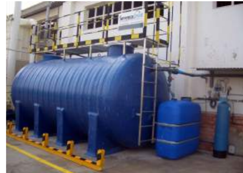
Industrial wastewater treatment plant. Flow 16 m 3 /day.
