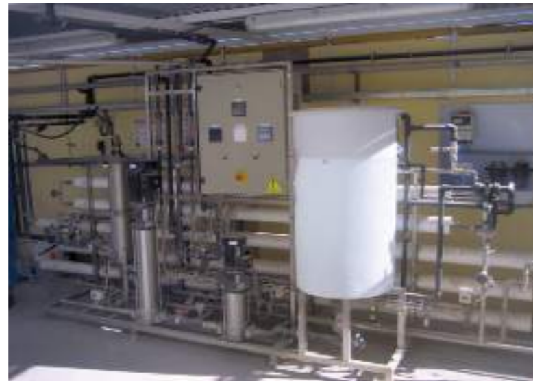
Two-stage reverse osmosis. Flow 25 m 3 /day.
