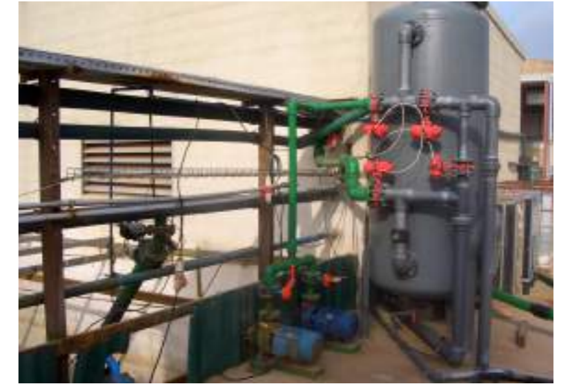
Pretreatment osmosis filter. Flow 100 m 3 /day.
